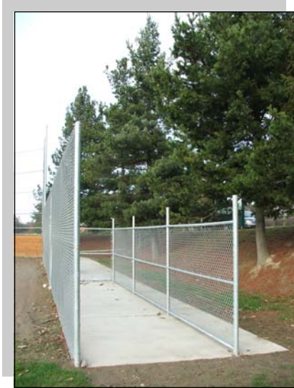
We still need materials and construction for four new first ever dugout roofs for Soundview Fields #3 and #4!
